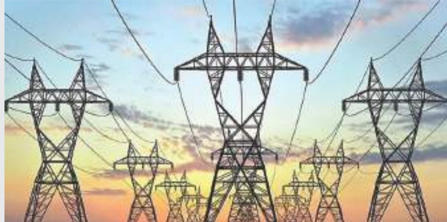
Grid-India in quarterly operational feedback 2025 also highlighted low voltages at 400kV Amargarh, Wagoora and Wanpoh
