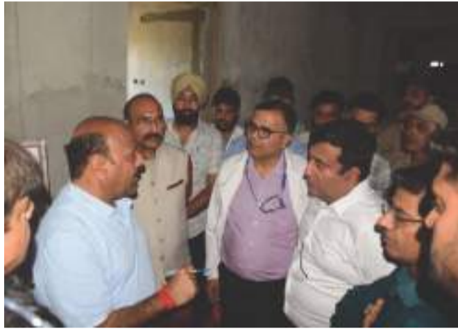
Ayurvedic Medical College, Sangani, Akhnoor, where he reviewed the ongoing hostel construction works along with MLA Akhnoor, Mohan Lal Bhagat.
