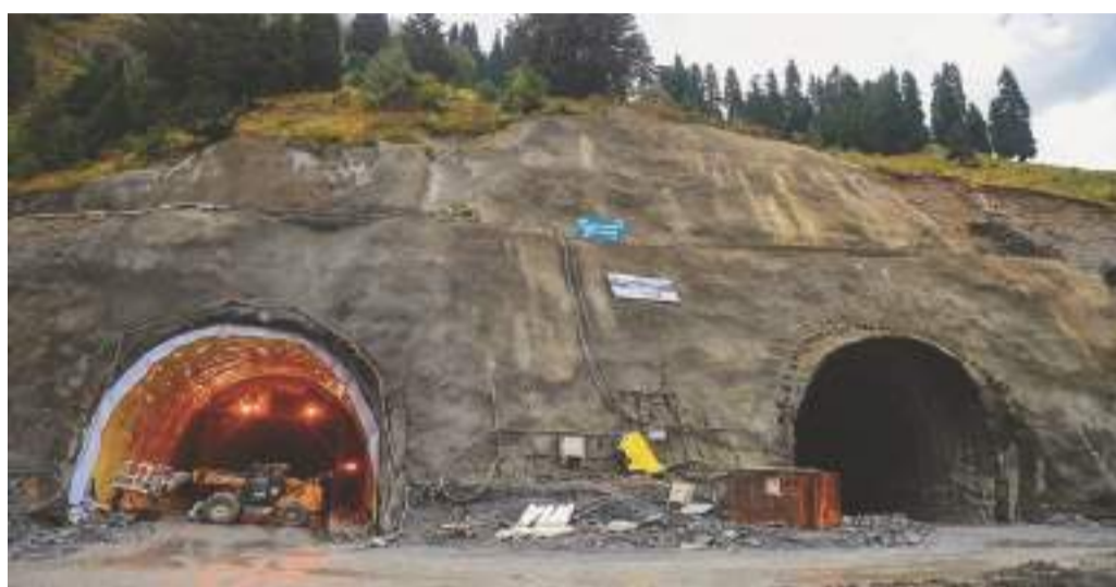
to the key tunnelling milestone where excavation faces from both ends meet.
